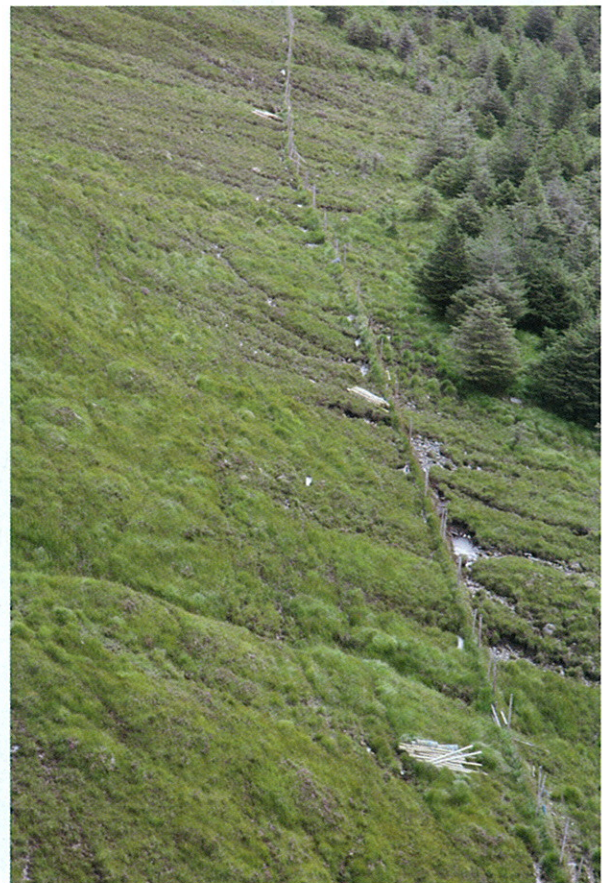
Fence bundles placed every 100m next to the old fence being replaced.
